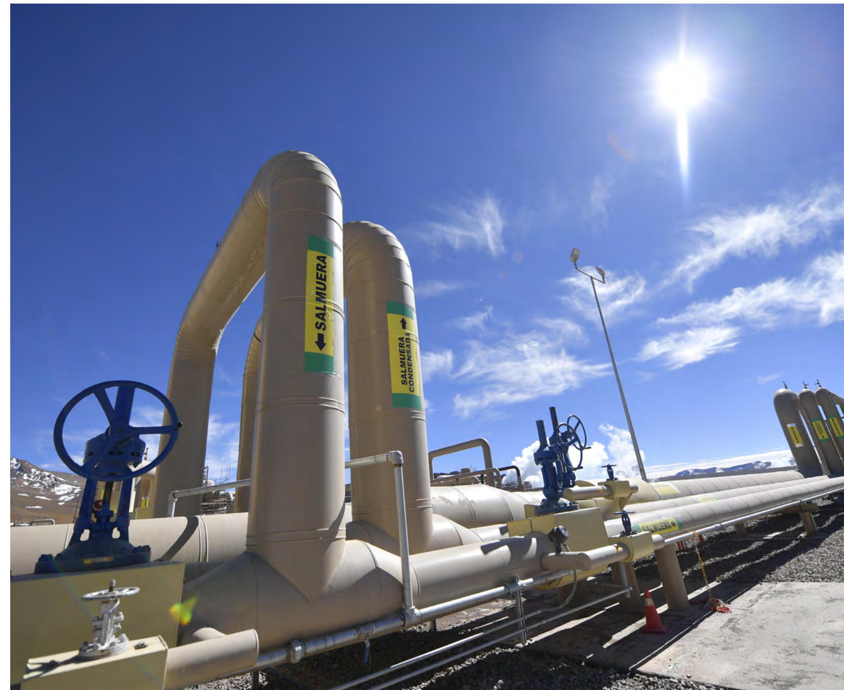
Cerro Pabellón geothermal plant. Enel Chile
