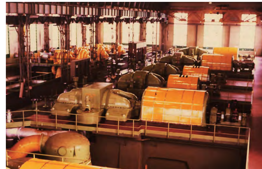
Interior of the Larderello 3 power plant (ca. 1970). Geothermal Museum of Larderello (Italy).
