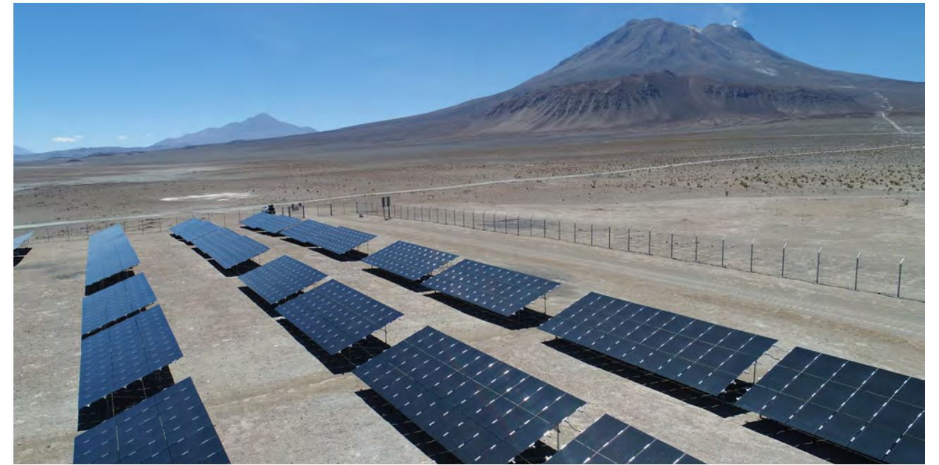
Photovoltaic panels at Cerro Pabellón camp. Enel (Chile).
